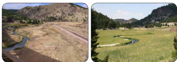
RESTORATION IN SILVER BOW CREEK'S DURANT CANYON WHERE IN SOME PLACES UP TO 21' OF MINE WASTE WAS REMOVED FROM THE STREAM BED AND BANKS. IN THIS AREA, SILVER BOW CREEK (FISH AND ALL) WAS DIVERTED INTO A 42" PVC PIPE FOR MONTHS AT A TIME.
