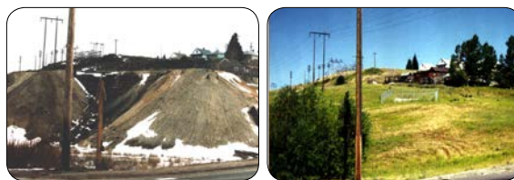
EXAMPLE OF REMEDIATION - "WASTE IN PLACE" - AT THE BUFFALO DUMP. REMEDIATED SITES ARE COVERED WITH 12"-18" OF SOIL CAP AND REVEGETATED.
