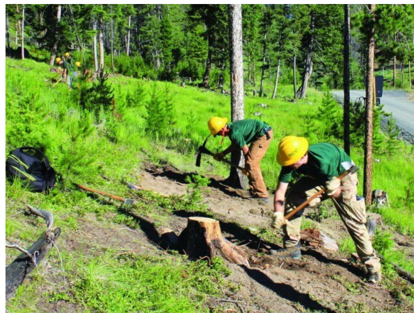
Montana Conservation Corps (MCC) builds new trails in Thompson Park. Photo courtesy of The Montana Standard .
