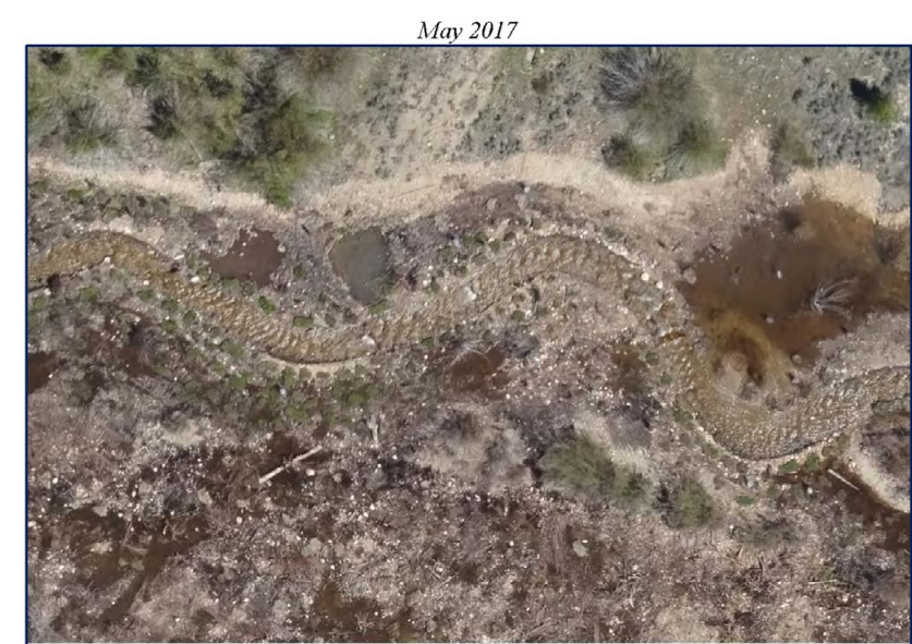
A new stream channel designed to regularly spill out of its banks.
